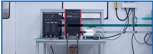
Switching Power Supply Testing Platform
